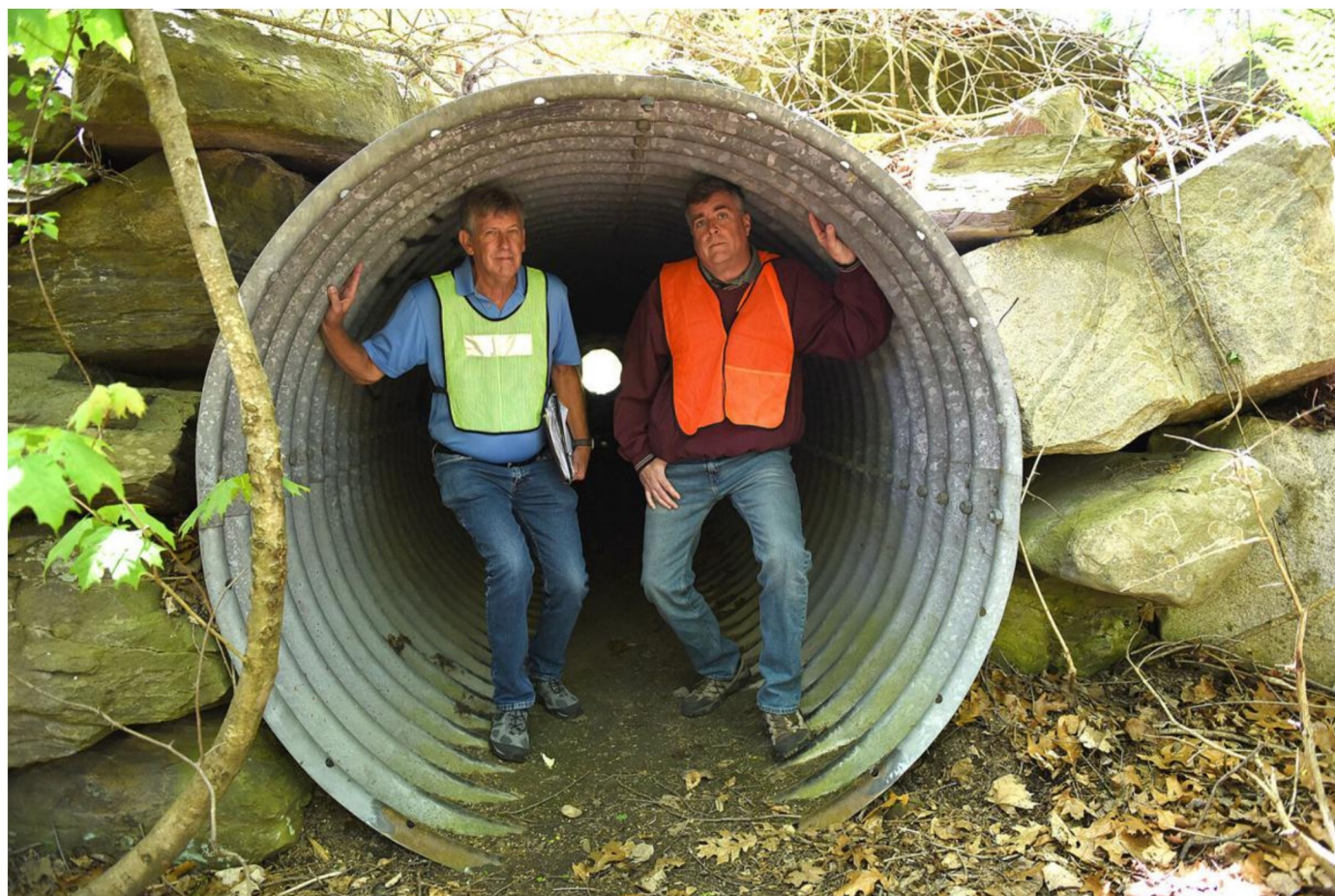
Derry Rail Trail supporters Alex Vogt, left, and Mark Connors stand in a culvert under Madden Road near where they want a tunnel for the trail to pass under a planned six-lane access road to a new Interstate 93 Exit 4A.
